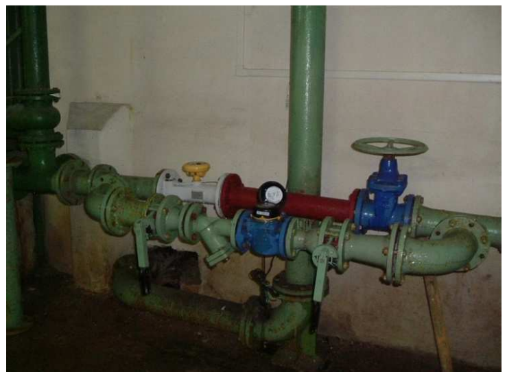
Measurement of industrial water
