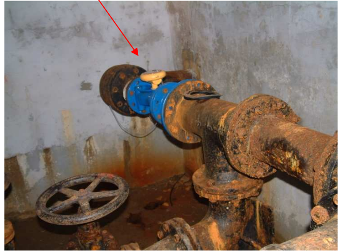
Measurement of drinking water in a station
