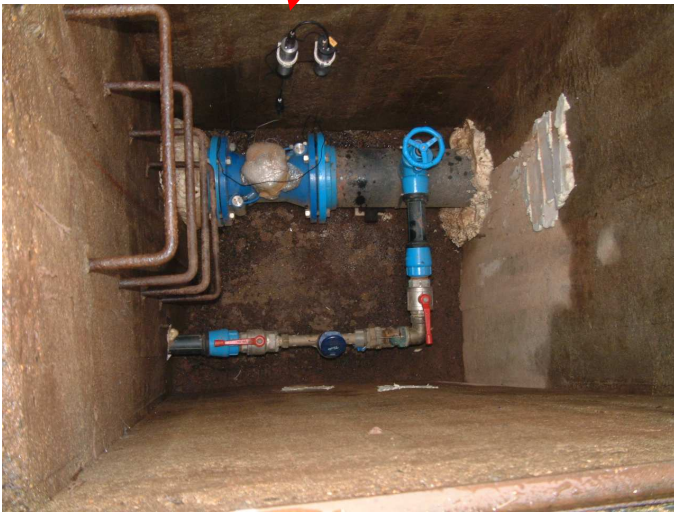
Measurement of drinking water in a chamber
