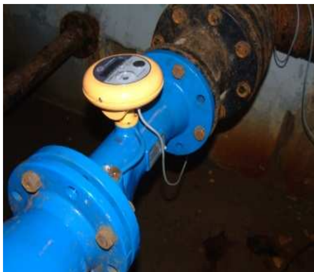
Measurement of industrial water
